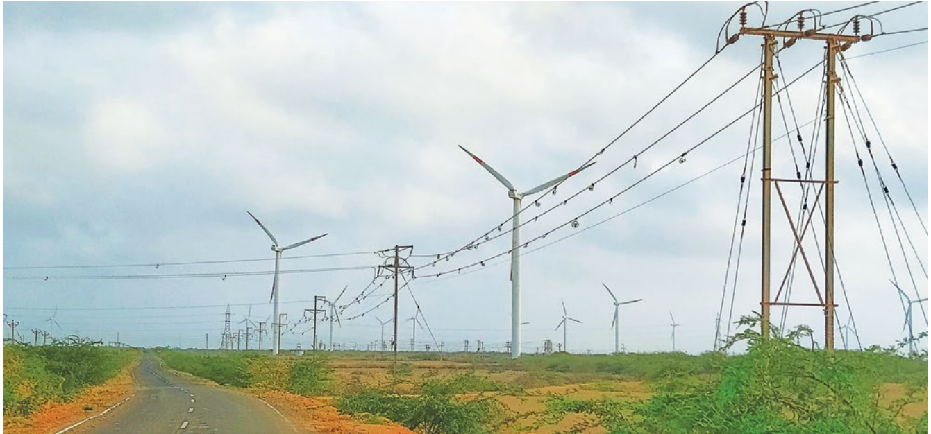
Bird diverters at ENEL Vayu at Abdasa Taluka, Kutch, Gujarat
