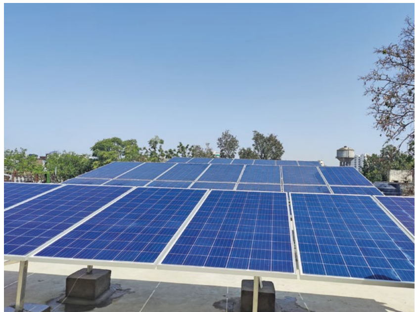
NIIF IFL has supported TAABAR to promote a holistic learning for students of a shelter home & school by enabling solar power generation
